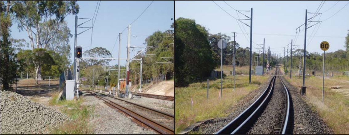
FIGURE 2: Signal LJ2 at Lytton Junction and, around the corner, entering the Fisherman Islands branch line
