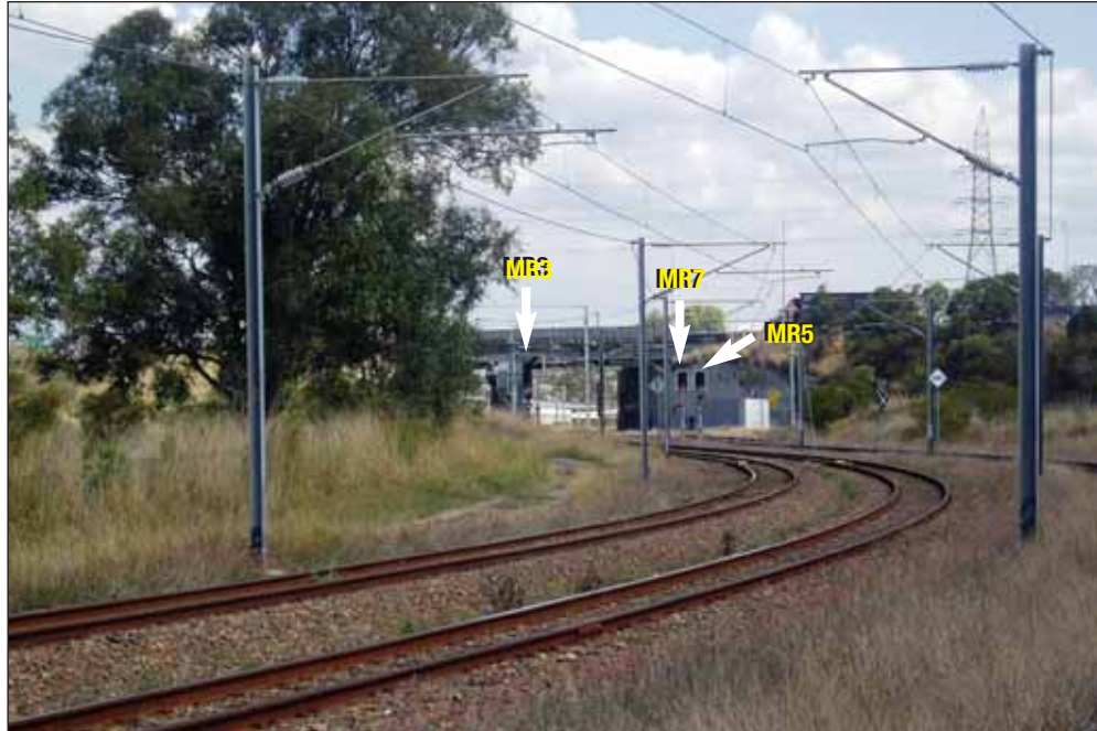
FIGURE 7: Aspect being displayed in signal MR5 visible 257.9 metres (daylight conditions)
