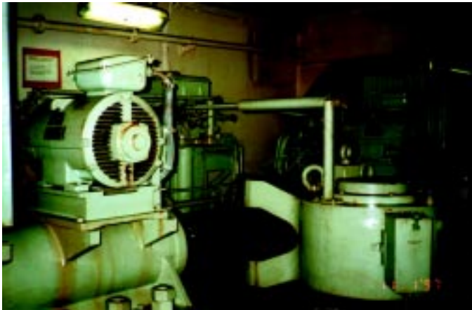
Tassos N steering gear showing port hydraulic ram, rudder stock, port and starboard steering motors and servo-control unit (centre background).
