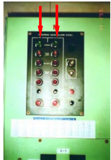
Bridge gear alarm panel showing green port and starboard steering motor indicator lights. (TOP)
