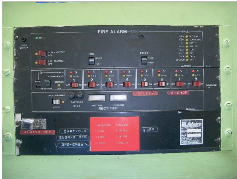
Figure 4: Bridge fire alarm control panel
