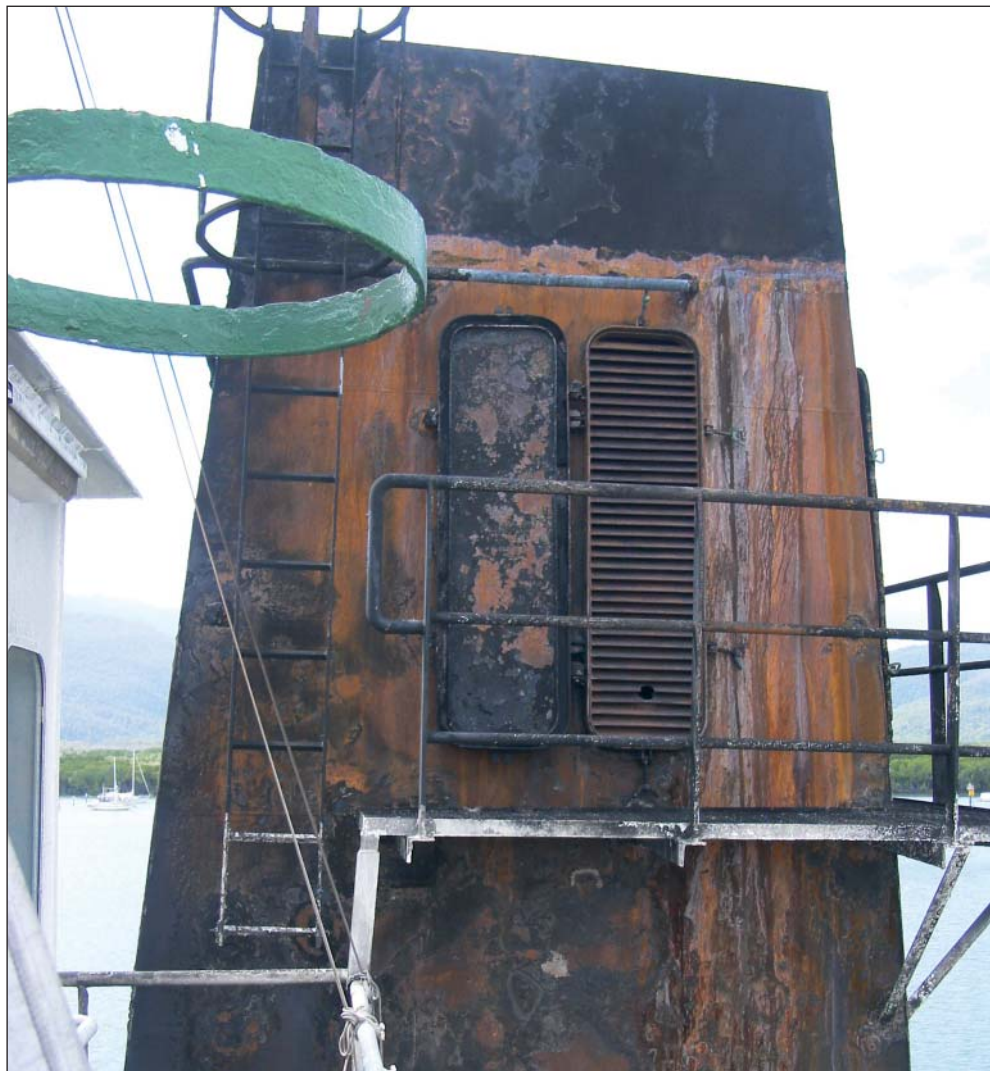
Figure 5: Funnel casing ventilation openings and closing dampers
