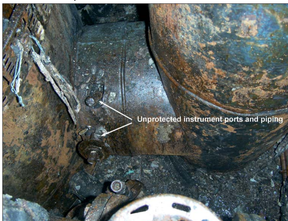
Figure 11: Oil-fired thermal fluid heater exhaust piping indicating the unprotected instrument ports
