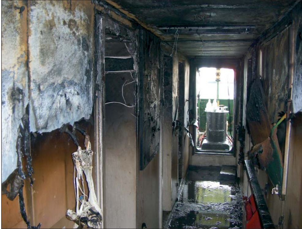
Figure 6: Damage to accommodation alley way
