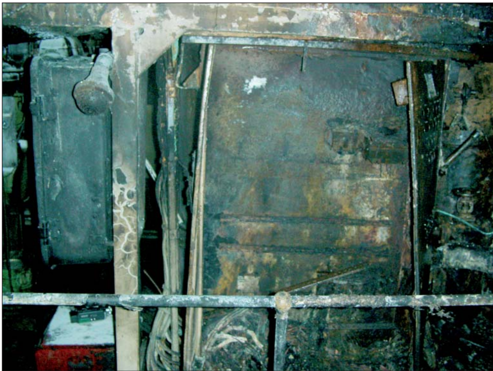
Figure 7: The remains of the oil-fired thermal fluid heater control cabinet
