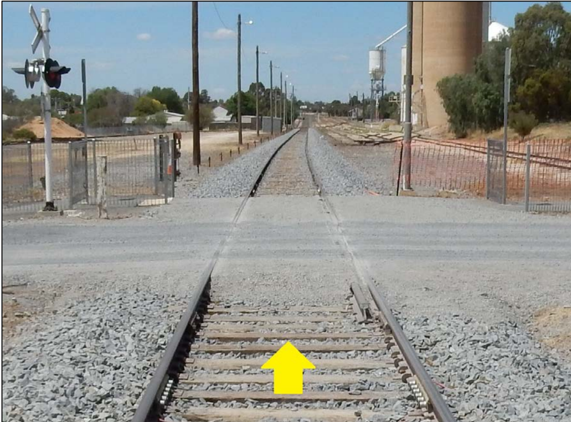
Figure 7: The William Street level crossing after reinstatement, similar in construction to the pre-derailment installation except timber sleepers used instead of concrete.
