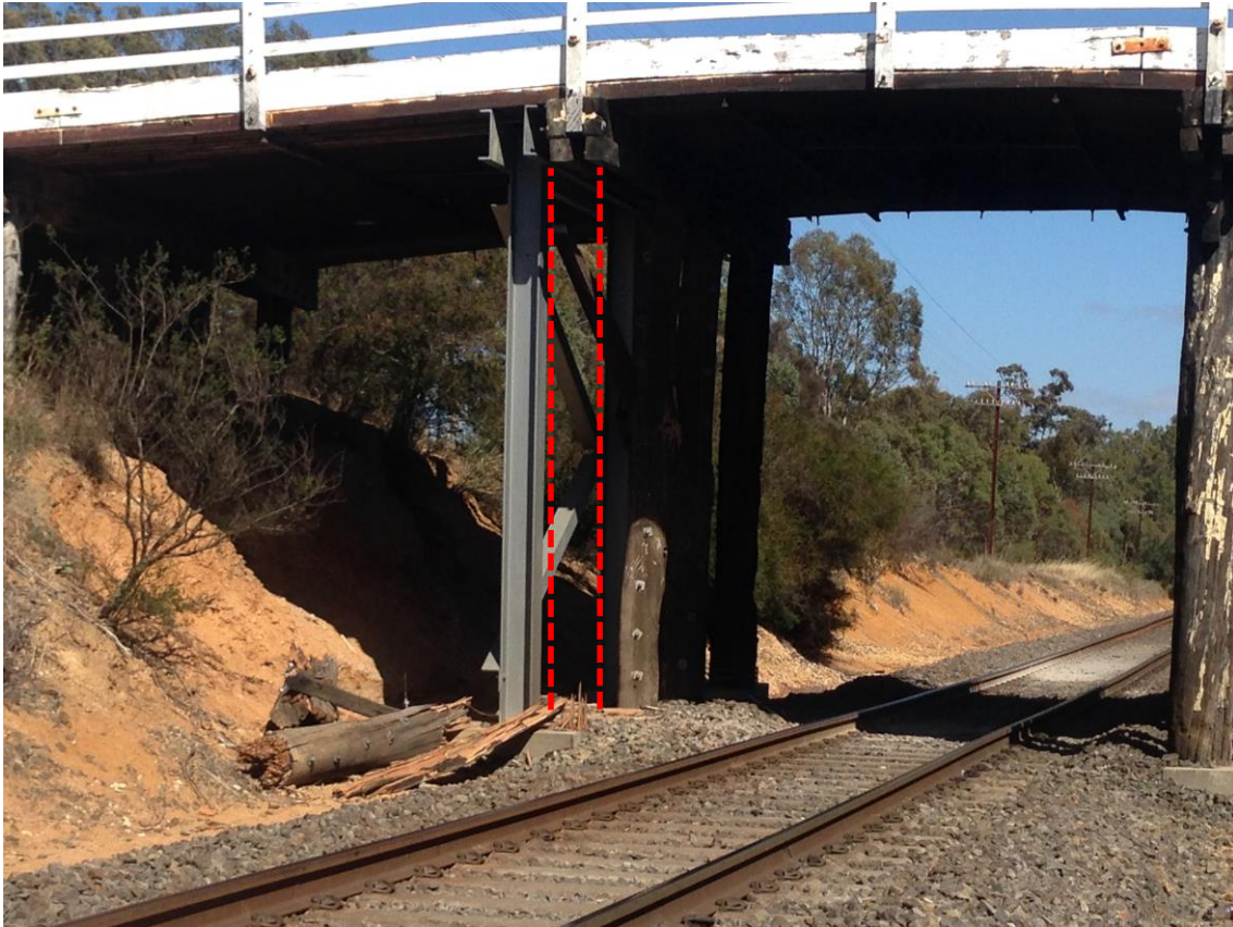
Figure 2: Paxton Street bridge damage
