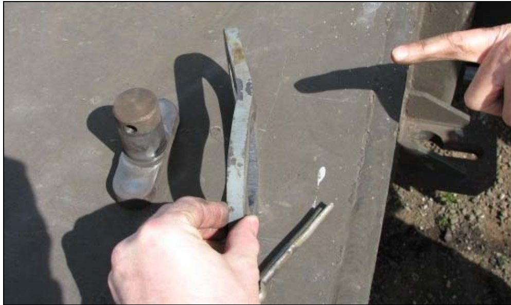
Figure 15: Retainer pin, distorted anti-wear collar and split pin inspected on site
