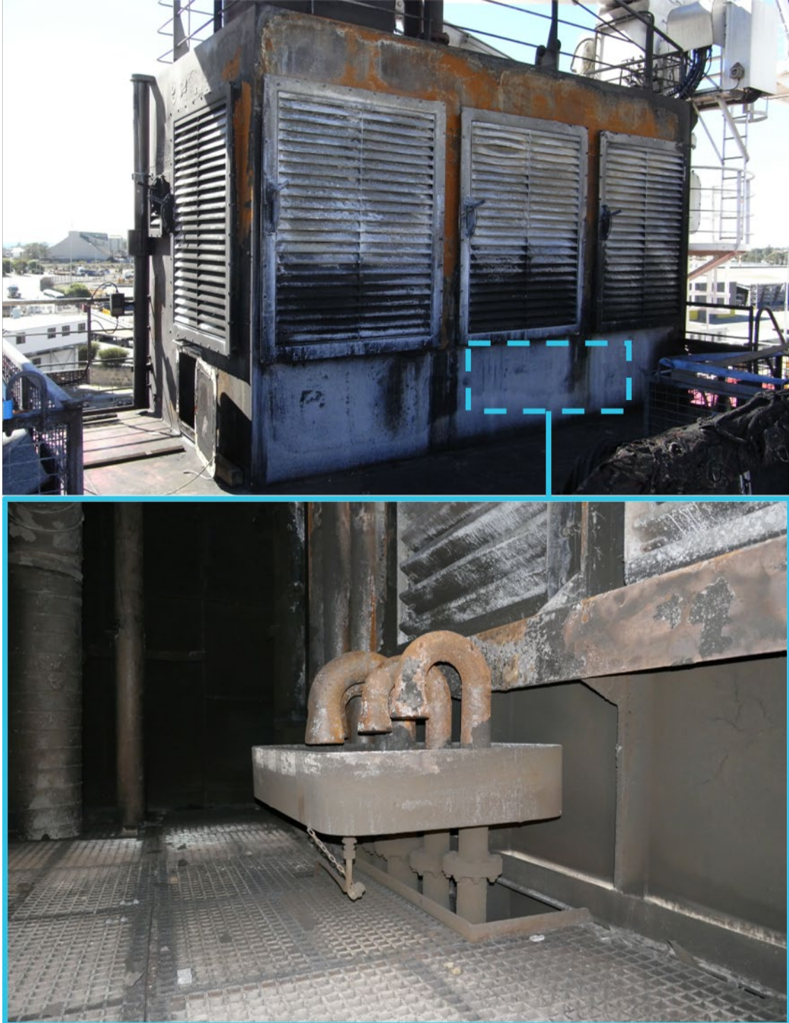
Figure 7: Port engine room exhaust casing (inset photo: close up of internal vent pipes)
