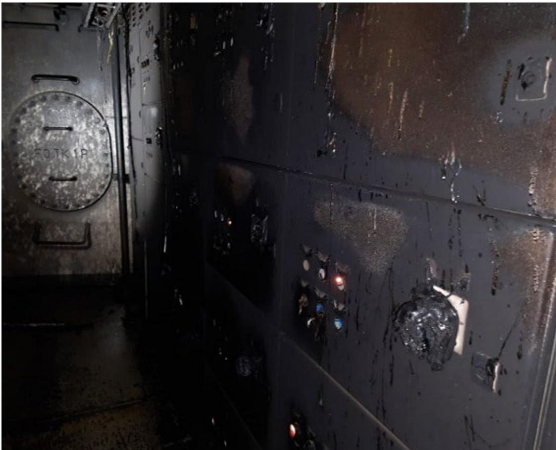
Figure 6: Fire damage inside the port engine room
