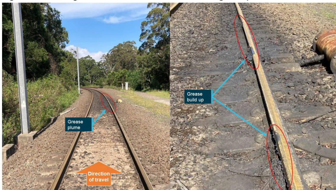
Figure 12: Rail flange lubrication device at 97.030 km and grease plume
