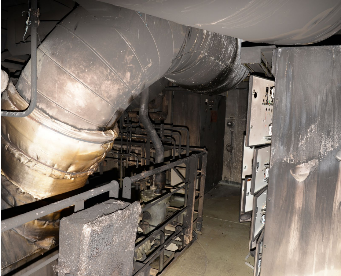
Figure 8: Fire damage inside the port engine room
