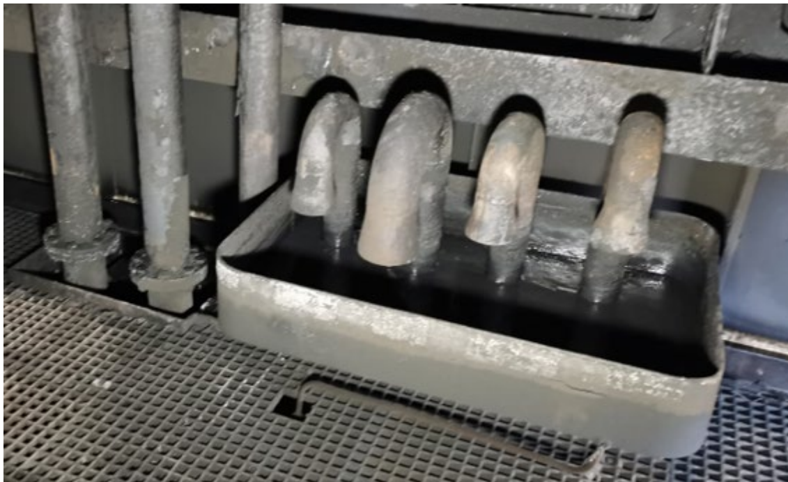
Figure 10: Fuel in port settling tank air pipe save-all
