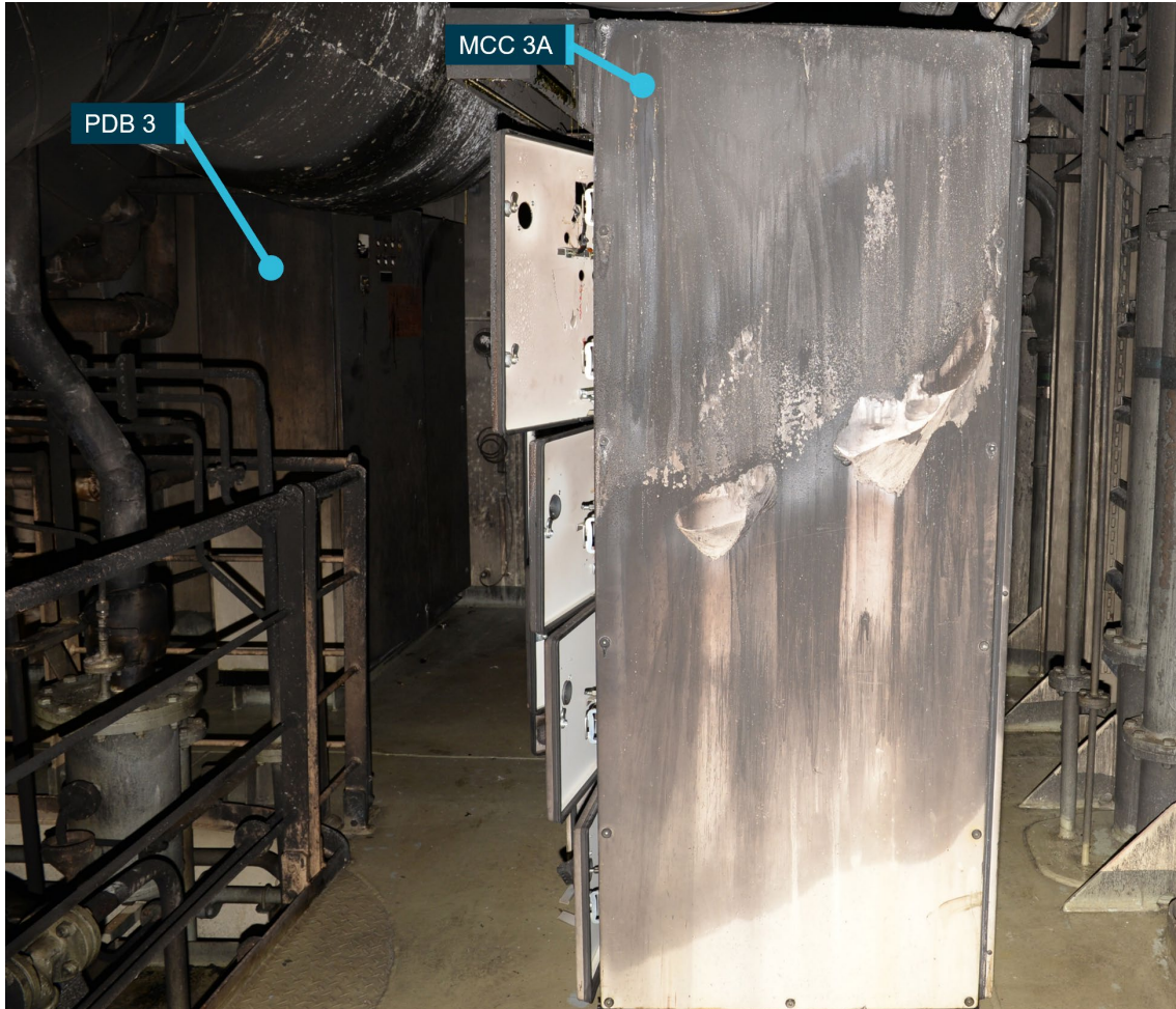
Figure 20: Electrical enclosures at forward end of B-Deck
