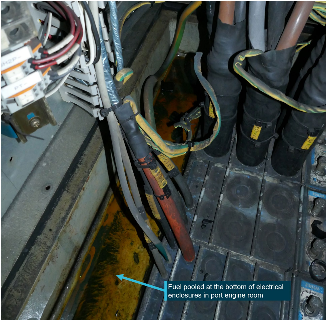
Figure 28: Fuel pooled inside electrical enclosures on B-Deck in the port engine room
