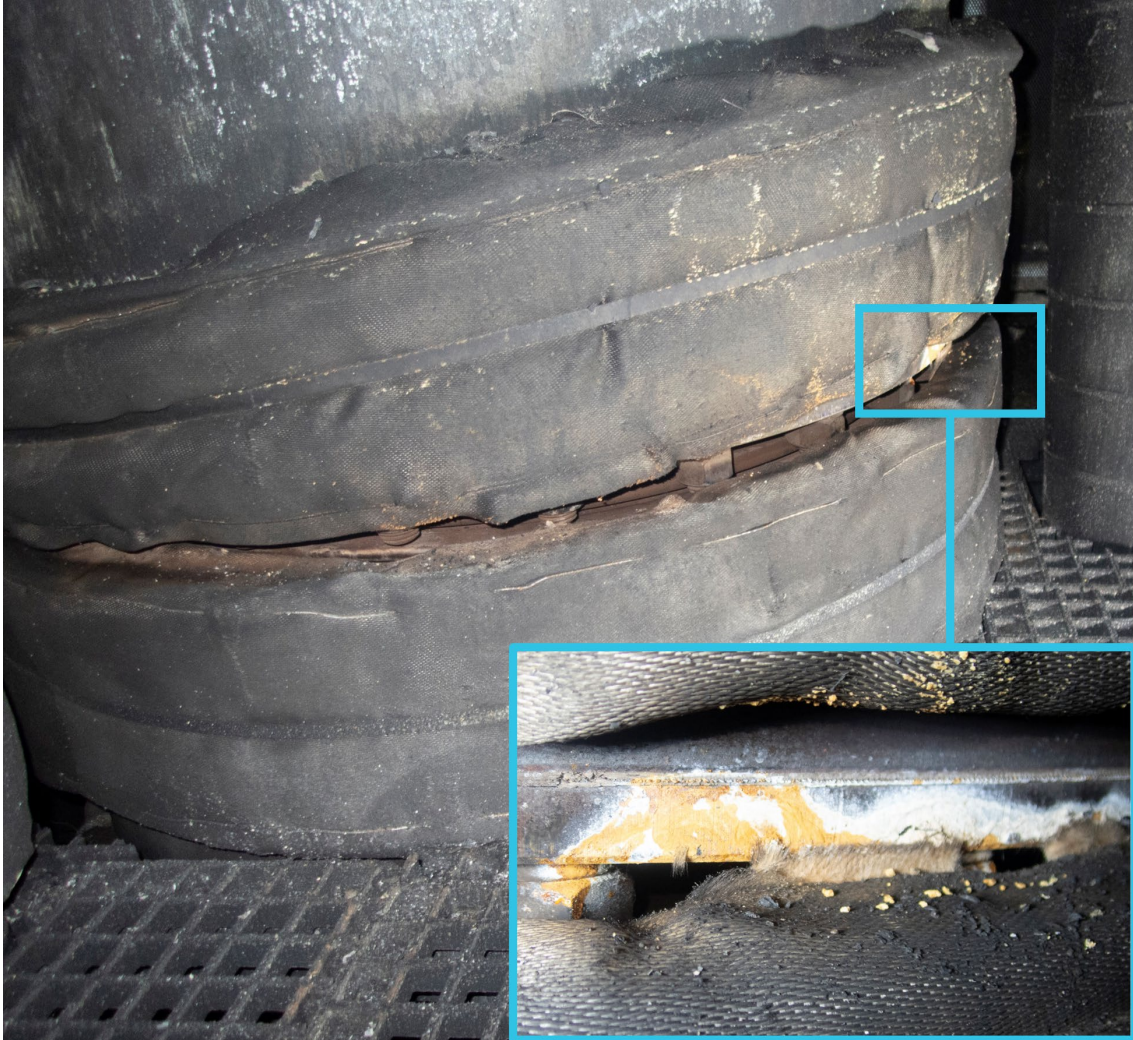
Figure 21: Gap in sections of insulation on exhaust trunking of DG3
