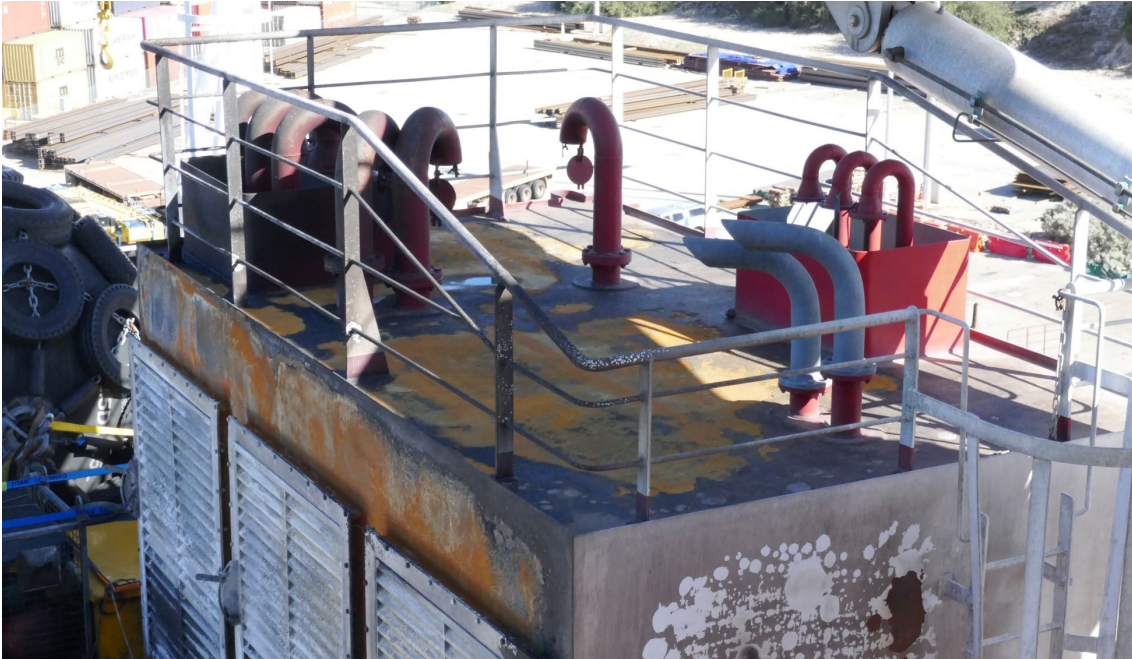
Figure 24: Top of exhaust ventilation casing
