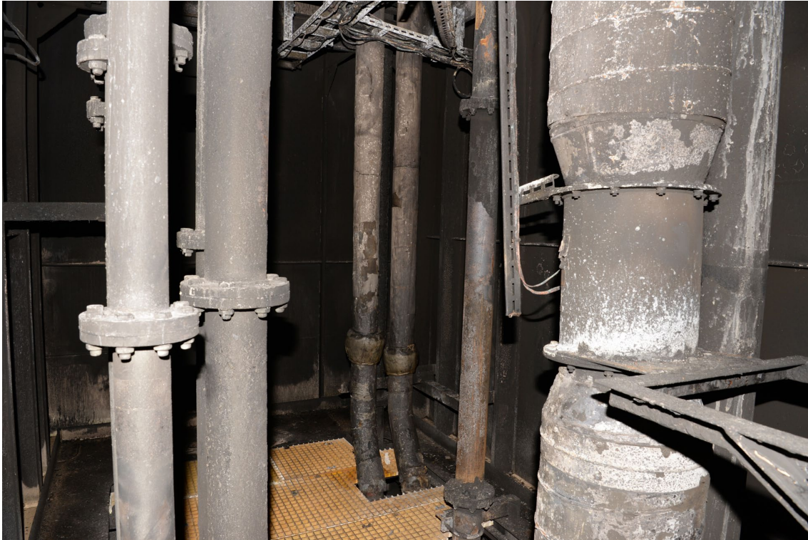
FRP grating deck replaced on board prior to investigator access. Source: ATSB
