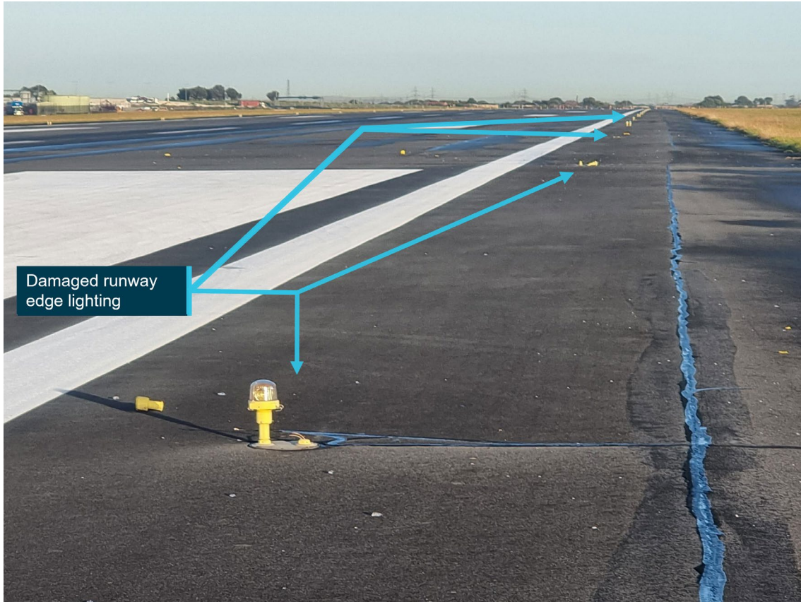
Figure 2: Damaged runway lights
