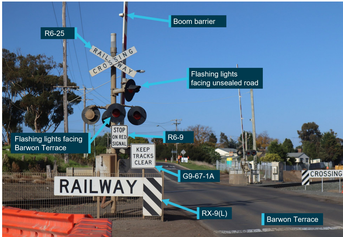
Figure 4 - Level crossing protection equipment at the Barwon Terrace level crossing
