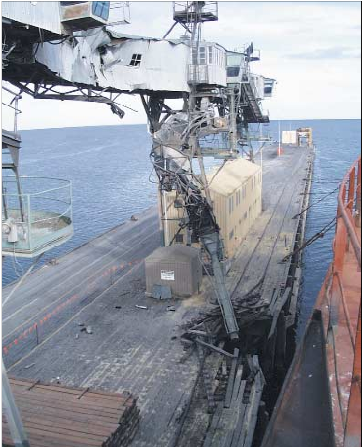
FIGURE 3 Wallaroo jetty and grain loader damage
