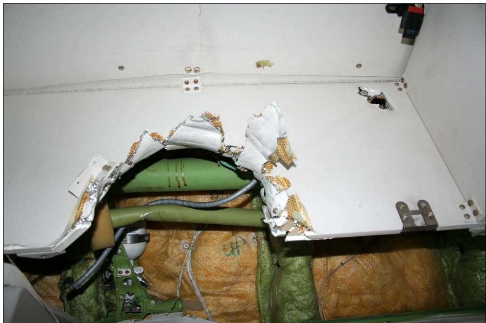
Figure 26: Semi-circular damage in partition of compartment above R2 door
