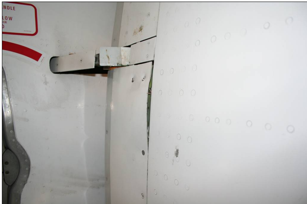
Figure 17: Cabin R2 door – damage to external panelling
