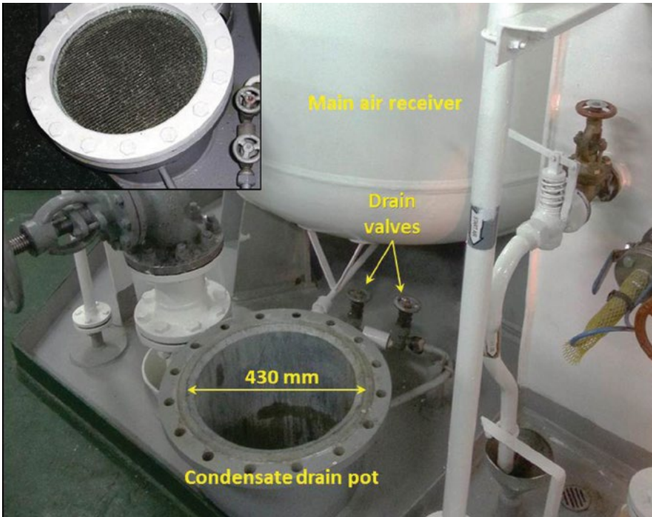
Figure 3: Main air receiver condensate drainage pot arrangement on board Nireas with inset showing the observation glass in place
